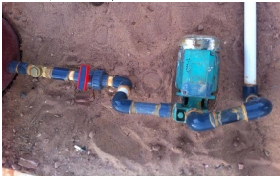
Fig. (4) Pumping unit including (AC) motor pump.
