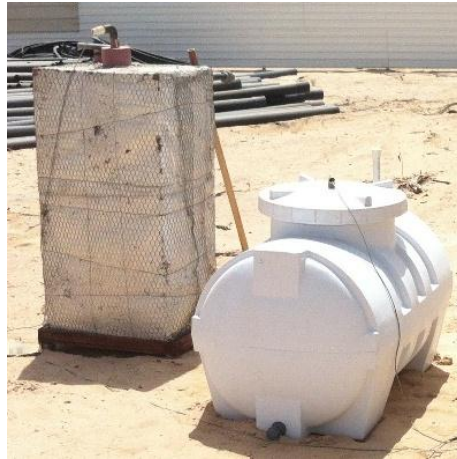
Fig. (12): Two water storage tanks of two different materials (polycon and insulated steel tanks)
