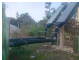
a- Two solar collectors for heating GH1
