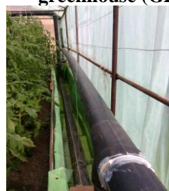
d- Right thermal storage tank
