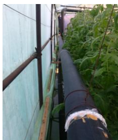
c- Left thermal storage tank
