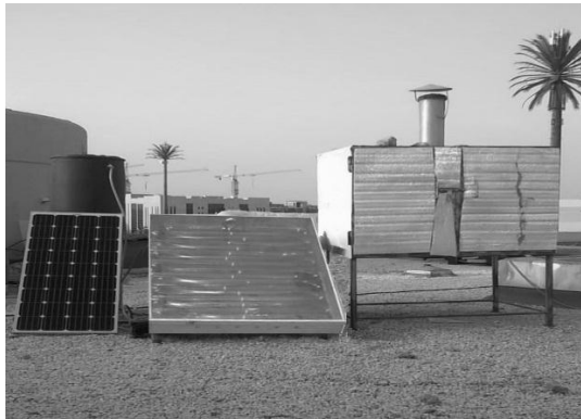
Fig. 1. The PV solar drying system.
