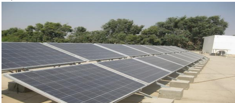
Figure (2): Solar panel generator.
