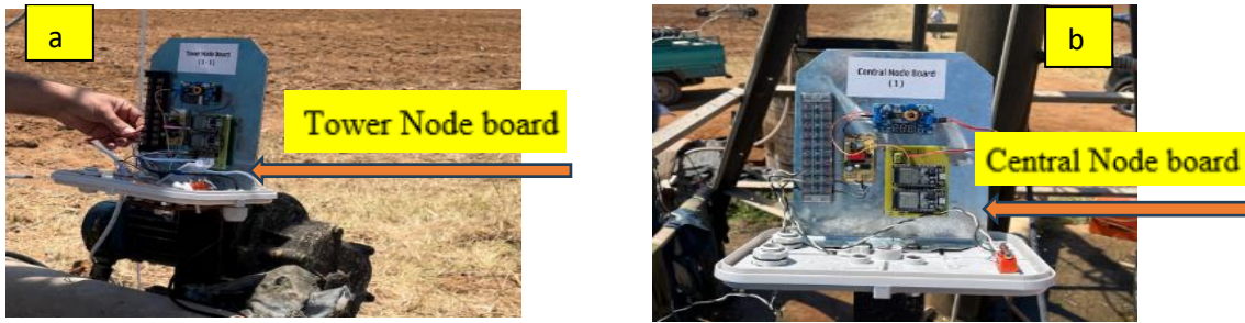
Figure (17): a-The tower node boards installation, b-The Central node board installation Data acquisition; and statistical analysis
