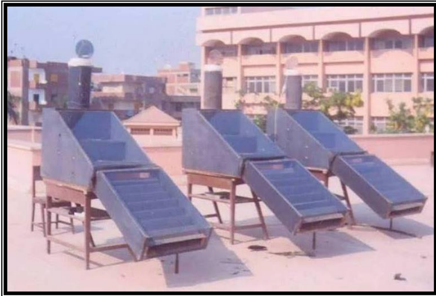
Fig. (2 )Solar drying systems.
